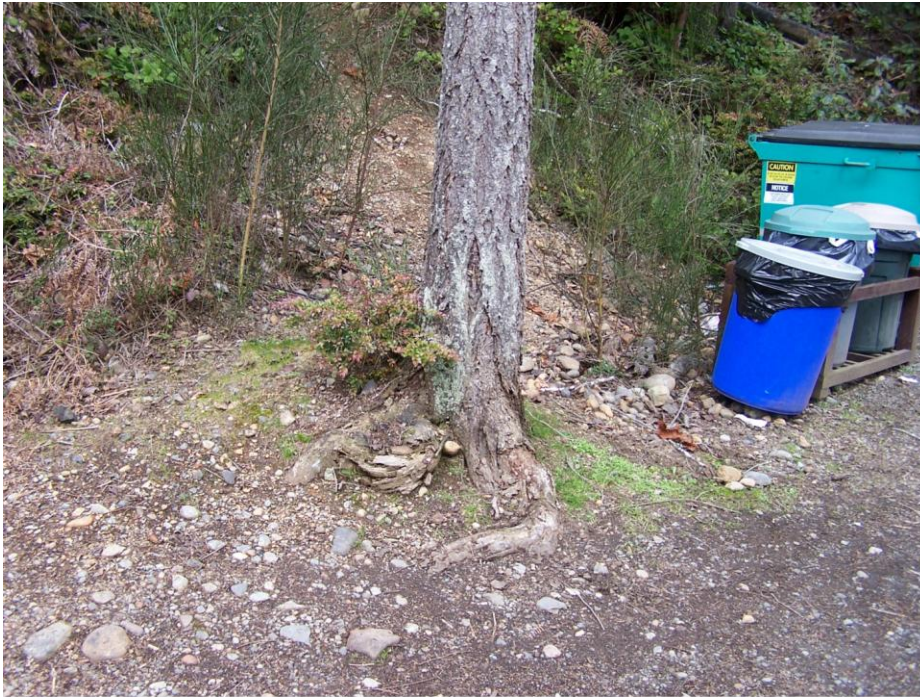
Figure 07 Image #2704 / Mechanical root damage at road edge in Marina Commercial area / Photo: RMG
