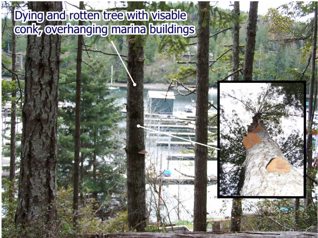
Figure 04 – Image #2744 & 2747 / Heart rot tree overhanging Marina buildings and service area / Photo: RMG
